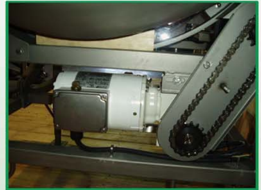
WASHDOWN MOTOR AND GEARBOX
